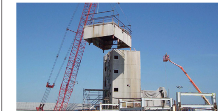
Building 143 at NECD, the site of the final step in the VX production process, was demolished in March 2006.
