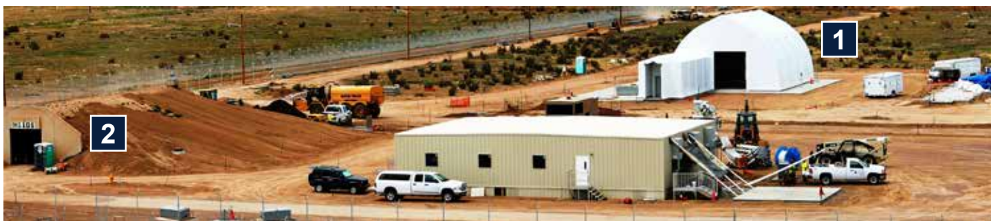
Construction of the PCAPP EDS began in early 2014. The sites included two environmental enclosures (1) for the EDS and the permitting of igloos (2) to safely store the munitions pending destruction.
