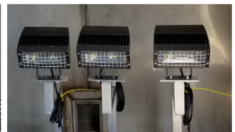
Light fixtures, switches, outlets and air conditioning units must meet strict non-explosive design requirements to reduce the risk of fire in the IHF.
