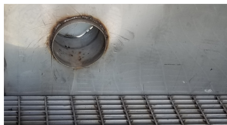
The IHF design includes a secondary containment area below the floor that would contain liquids in the event of a leak.
