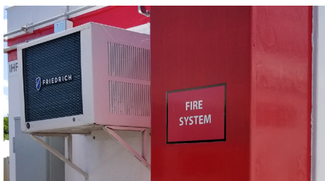
The IHF is equipped with an automatic fire suppression system in compliance with federal hazardous waste management regulations.
